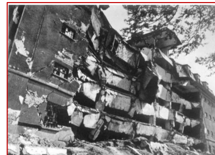
Fig. 6. Pancake failure of tobacco factory masonry building in central part of Skopje
