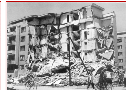
Fig. 5. Failure of right side structural unit of five story apartment masonry building in the West side
