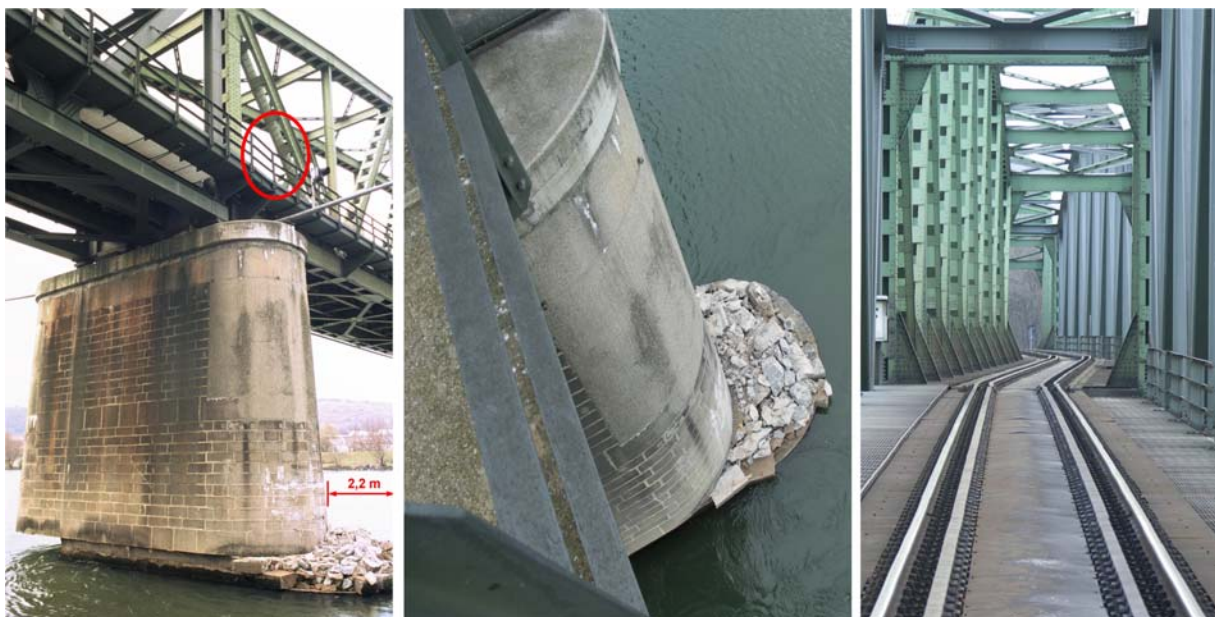
Fig. 4. Ship impact at a main pier of a railway bridge crossing the river Danube. Toe zone of the pier sheared off by 2.2 m; steel girders show multiple buckling.
